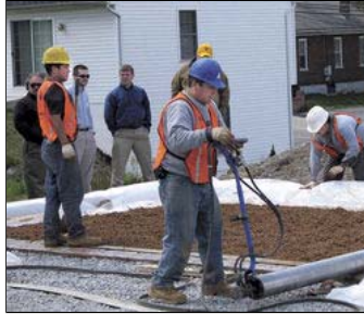
Construction workers lay pervious concrete Thursday outside of Potomac Construction Industries in Martinsburg. The demonstration was meant to educate engineers, developers and government officials about the benefits of the environmentally friendly building material, which captures storm water and allows it to absorb into the ground. (Journal photo by Christina Marnik)
